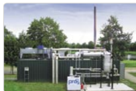
Biogas plant with gas cleaning station in Kleinbautzen, Germany
