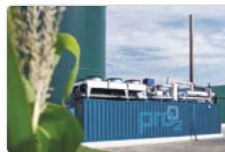
Biogas plant in Steinfurt, Germany
